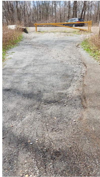
Figure 14 Airline Trail looking southwest towards Cook Hill Road. The trail surface is eroding due to stormwater
